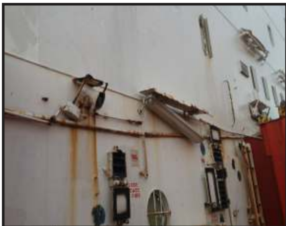
Light shades damaged on decks
