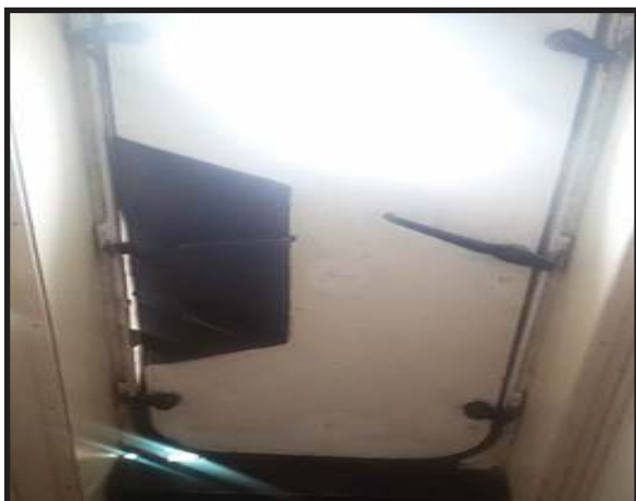
Accommodation Entrance door holed
